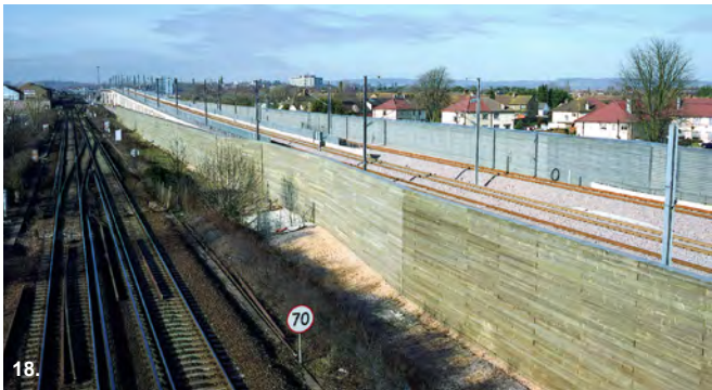
Acoustic fences were installed along the route to provide noise mitigation
