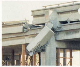
1. Failure of Cypress Viaduct, Oakland, 1989.
