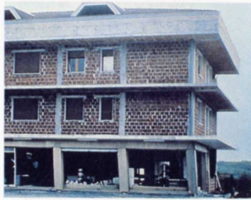
5. 'Soft storey' building which was damaged in the 1976 Friuli earthquake, and collapsed in an aftershock.
