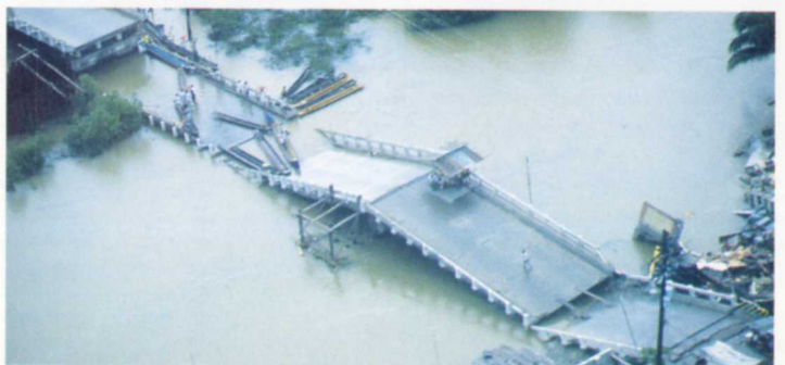
10. Liquefaction-induced bridge failure, Philippines 1990.
