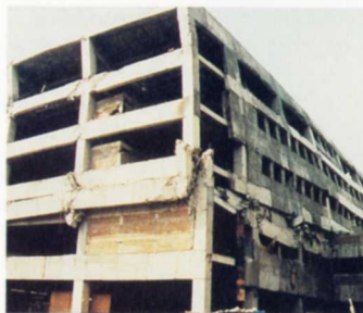
8. Column failures in the 1985 Mexican earthquake.
