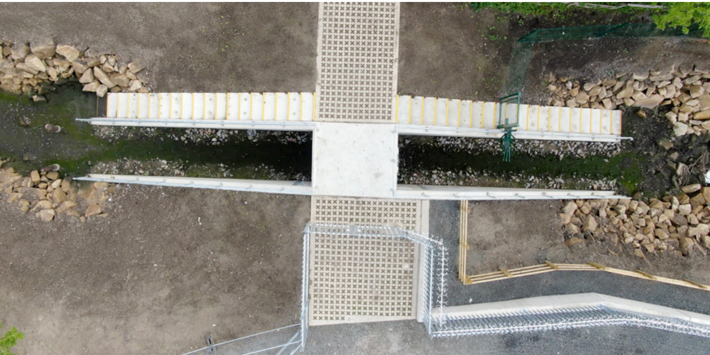
17: An aerial view of the concrete trough used along the Skinnersburn tributary
