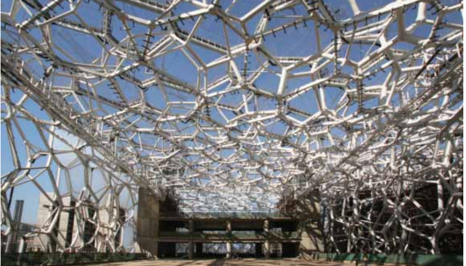
1. The structure of the Beijing Aquatics Centre (“Water Cube”): projects like this are now beyond conventional two-dimensional design and documentation methods.
