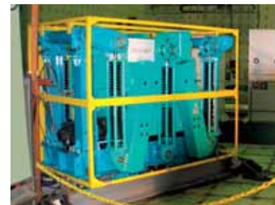
12. A 5 tonne active mass damper located at cab level.
