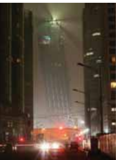
19. CCTV under construction at times presented almost surreal vistas from surrounding streets.
