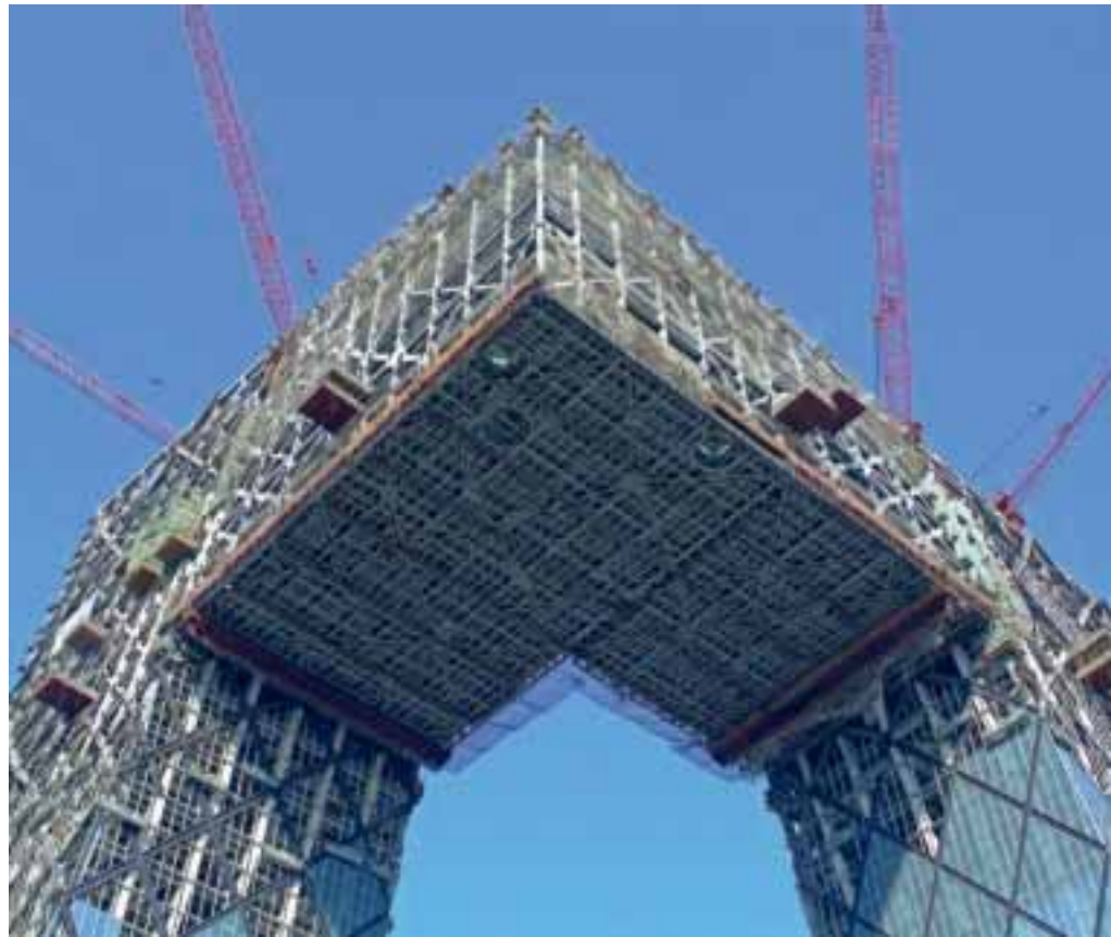
24. The completed Overhang structure, showing the three 3m diameter circles punched in the deck to create glazed viewing platforms for the public viewing gallery.
