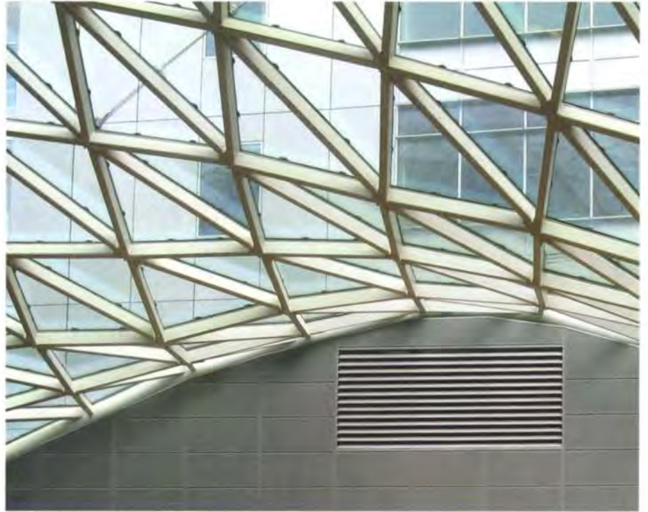
19. Perimeter smoke extract.
