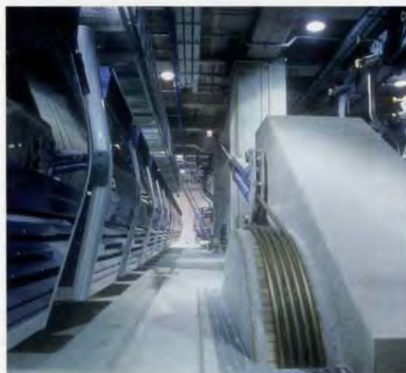
8. Anchor drum and cabin storage at Tung Chung terminal.
