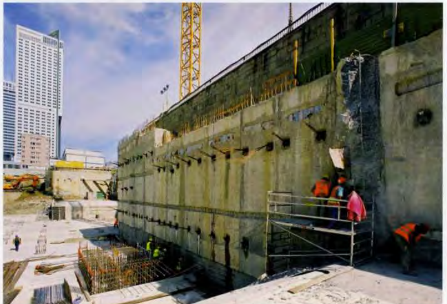
6. Diaphragm retaining wall with ground anchors, along the east edge of the site.
