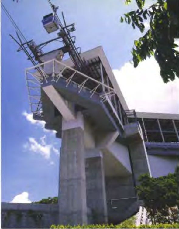
9. Structural support at the AIAS for cable catenaries leading to Tower 3 and on to Nei Lak Shan angle station (NLSAS).
