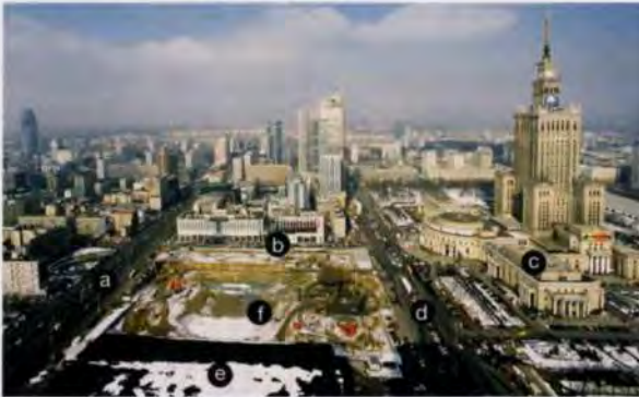
4. The site during basement excavation in April 2003: (a) Jana Pawła II Avenue, (b) Złota Street, (c) The Palace of Culture, (d) Emilii Plater Street, (e) Warsaw Central Railway Station, (f) Złote Tarasy.
