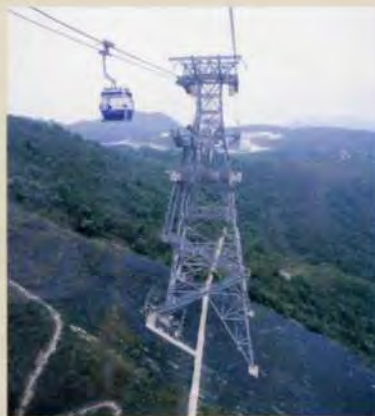
18. The completed Tower 7 showing the extent of slope stabilization, and the tower plinths.
