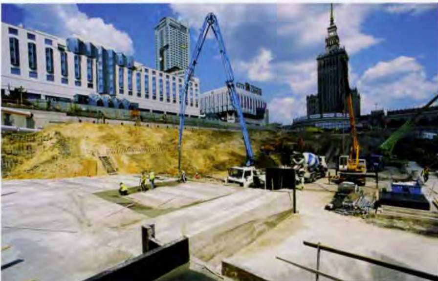
7. Raft foundation under construction at B4 level. On the left is the soil berm left in place to support the diaphragm wall along Złota Street, on the other side of which are the "City Center" shopping centre and the Holiday Inn Hotel.
