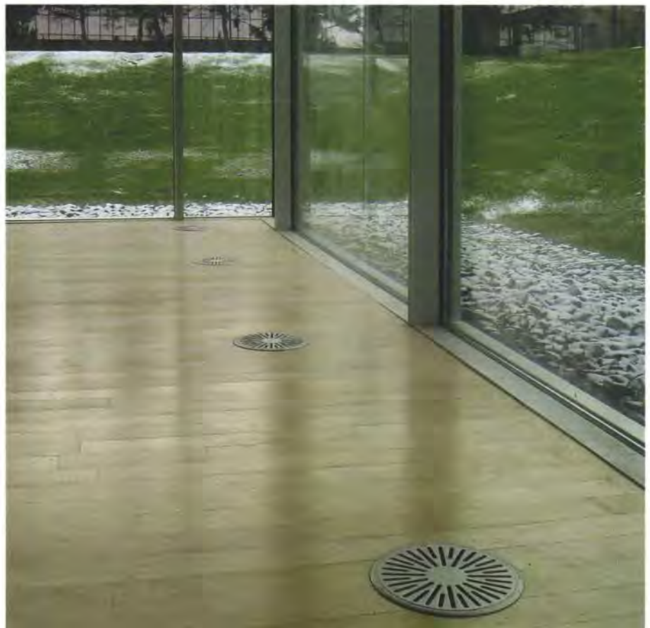
8. Swirl-type floor diffusers are ducted to the FPBs for the conference rooms to mitigate heat gains and losses.
