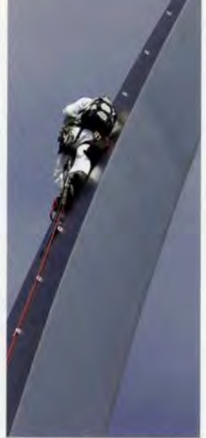
19. Abseiler near the tip of one of the spires. Ropes are attached to engineered clips welded to the back face of each spire to accommodate such access for future testing and inspection.
