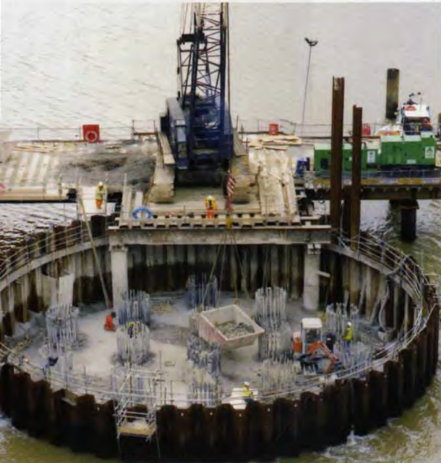
3. The river pier foundation: 1.8m diameter piles for the Medway Viaduct, formed after detailed vertical and lateral preliminary pile testing onshore.
