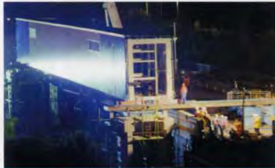
14. Thames Valley utility bridge, to carry Ford services, being lifted into place.
