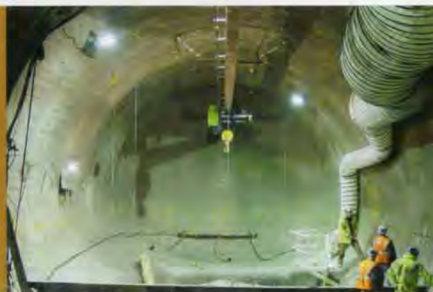
15, right: Ventilation adit at Corsica Street with sprayed concrete lining; running tunnel connection being constructed through invert.
