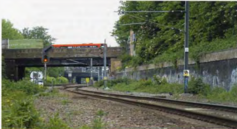
6. Infrastructure dating from the 19th century in poor repair, looking west at Cannonbury West Junction, with Cannonbury Station platform in the background.
