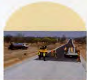
7. Surfacing unit with chip spreader about to lay the seal coat of 10mm stone.
