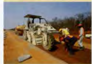
9. Cement stabilization using mechanical self-propelled reclaimer with water bower connected for moisture conditioning during mixing.
