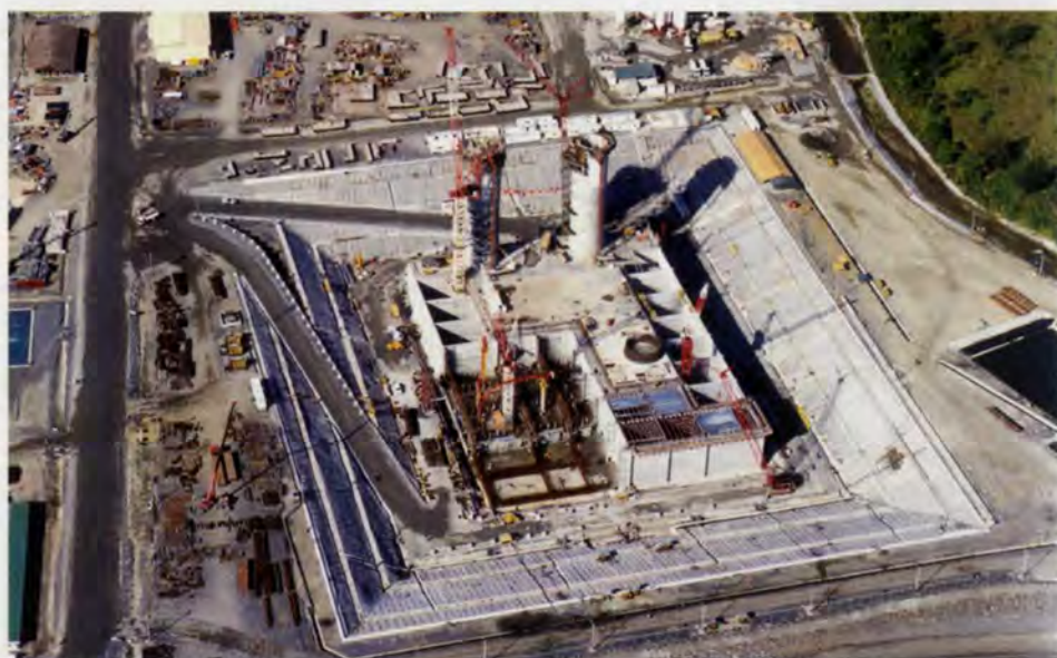
5. The CGS in the casting basin, with slipforming of the base caisson in progress.
