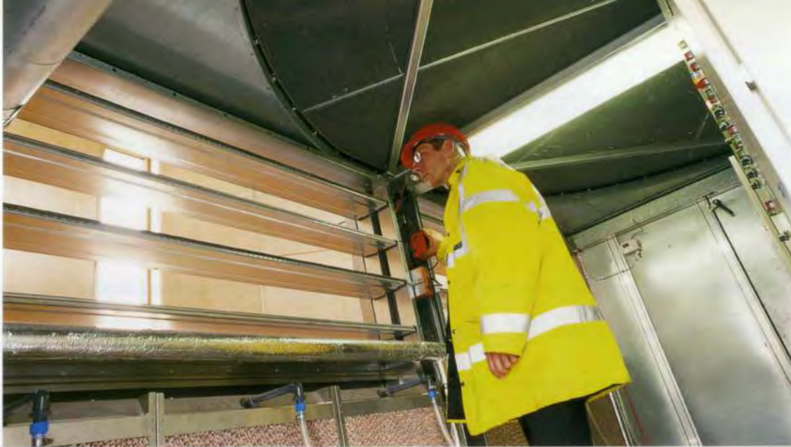
9. Interior of lower part of AHU, with engineer beneath thermal wheel, looking through bypass damper.
