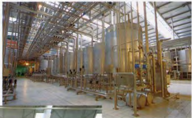
9. Interior of beer processing and brewhouse.
