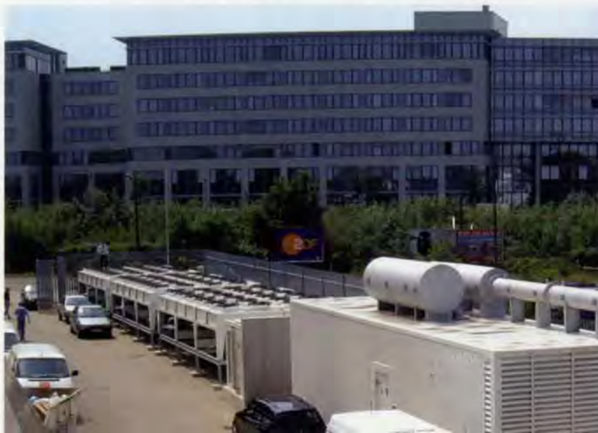
3. External plant at Düsseldorf datacentre.
