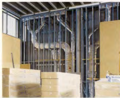
7. Air-conditioning ductwork being concealed behind thick walls.
