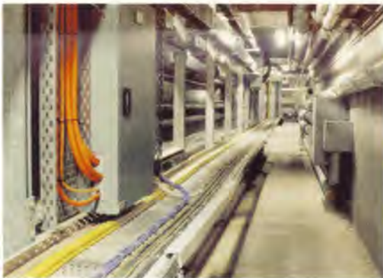
13. Typical transverse services tunnel beneath the exhibition floor.
