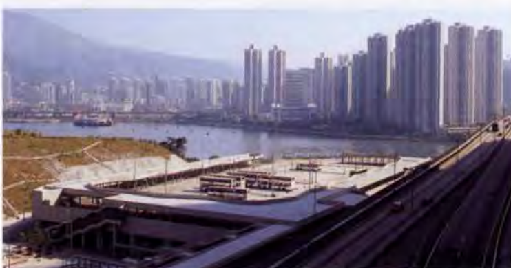
12. Public transport interchange under construction. Beyond is the district of Tsuen Wan across the Rambler Channel.
