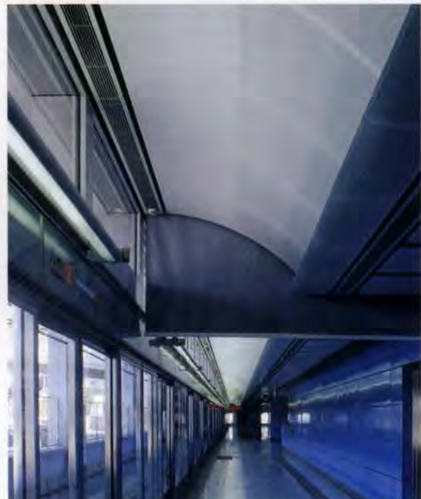
4 right: Half sound-absorptive curved panel and flat panel above the platform at Olympic Station.
