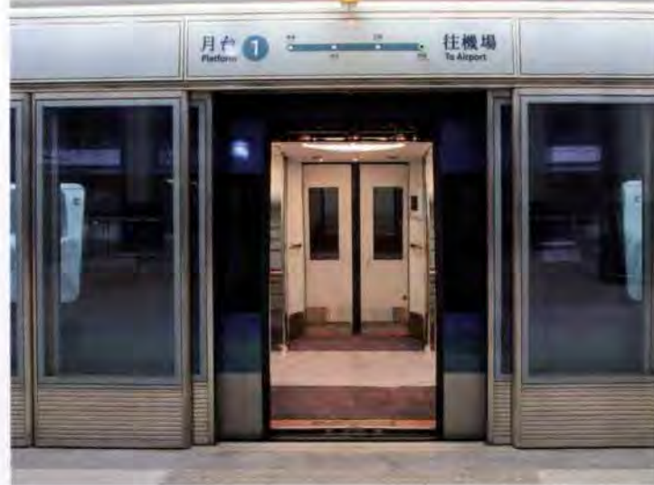
3. Screen doors open in front of stationary Airport Express train at Hong Kong Station.
