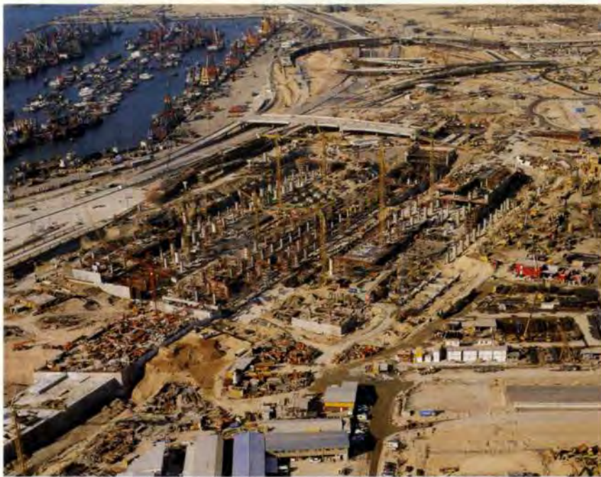
4. Station structure under construction, December 1996: south cut-and-cover tunnels on the left; north cut-and cover tunnels just beyond end of Station.
