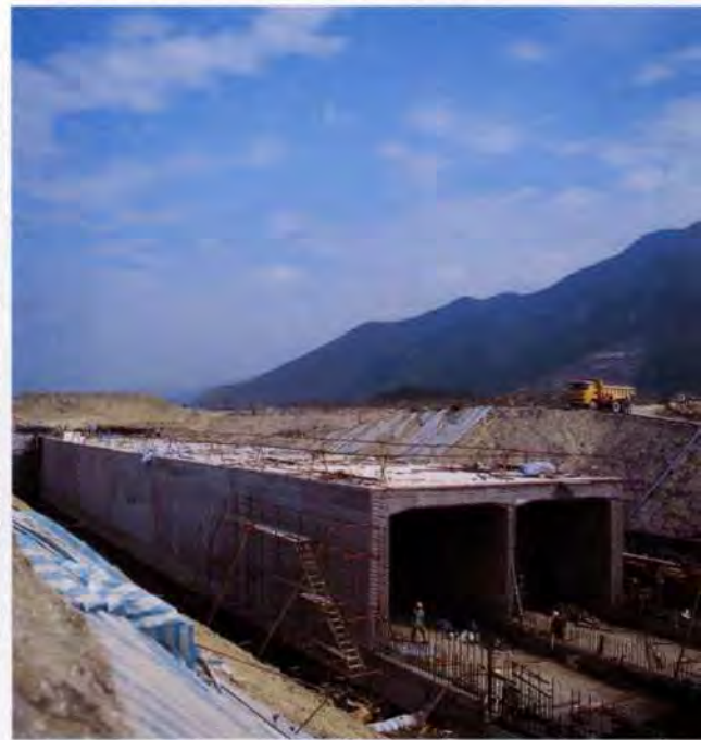
9. Twin box cut-and-cover running tunnels under construction in the new reclamation with the hinterland of Lantau Island behind.
