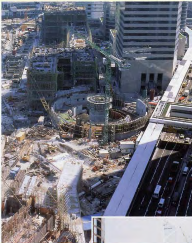
3. Construction from the west; centre: foundations of the International Finance Centre (South West Tower); behind: the Station buildings; right: Connaught Road Central.
