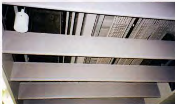
3. Baffle absorptive ceiling above the Tung Chung Line platform in Kowloon Station.
