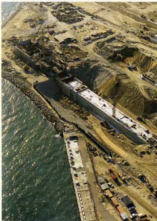
13. South cut-and-cover tunnels connected to KVB. The extreme closeness of both tunnels and KVB to the harbour is evident.
