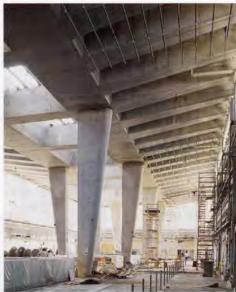
8 above Completed in situ concourse roof structure with acoustic ceiling framing under way.
