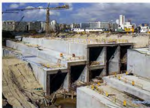
15: South cut-and-cover tunnels, showing multi-cellular nature of box, with 'stitching strip' gap. The Station is beyond, on the left.
