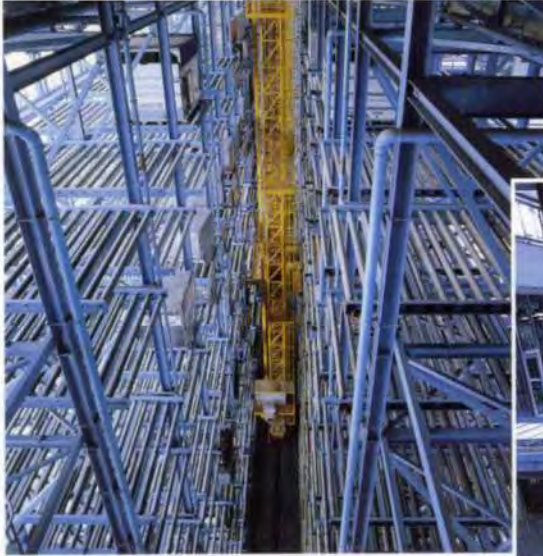
6. Stacker crane within void between CSS racking, from roof level.
