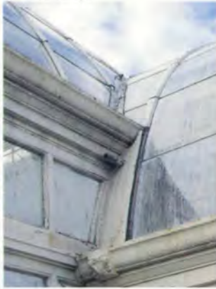
4 below. Typical deterioration of wood valleys.
