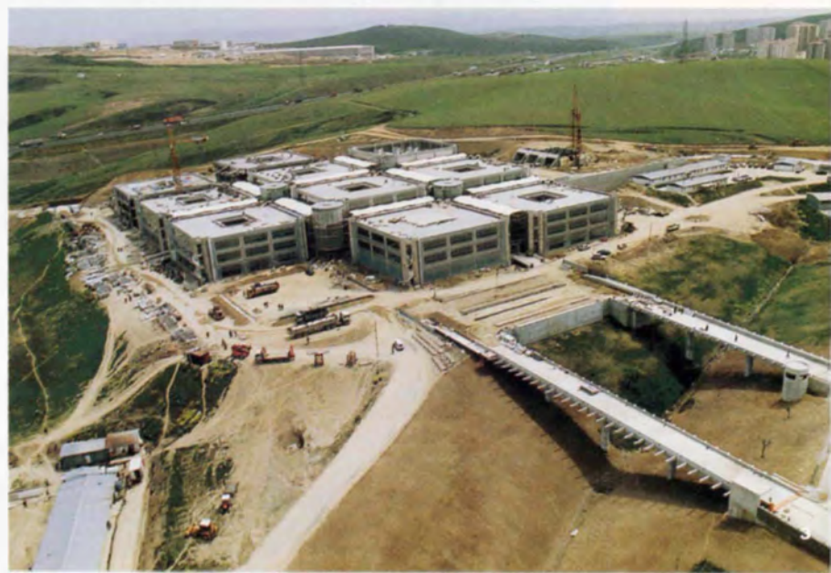
General view of construction site, September 1996, facing east. The two Phase 2 blocks are at the rear, with the motorway in the distance.
