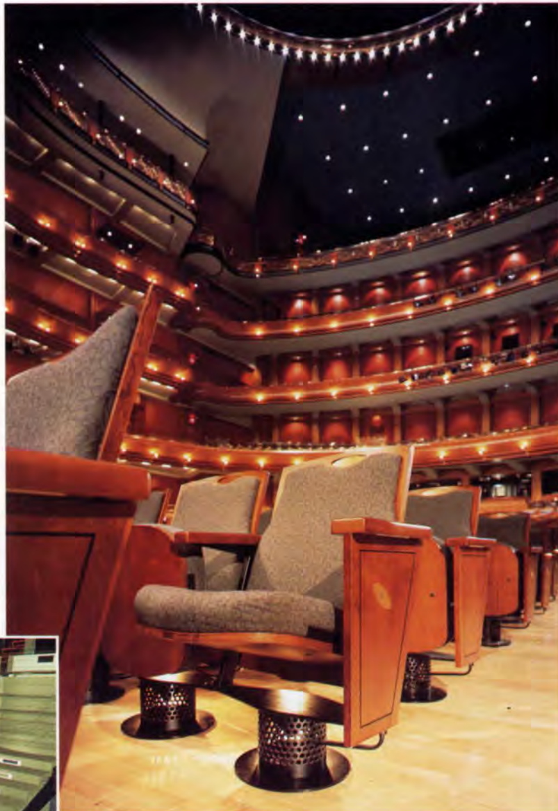
13. Underseat air distribution through Prudential Hall.
