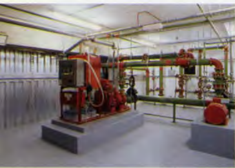
8. Water tank and pump set for sprinkler system.
