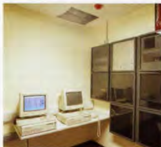
6. Main fire alarm control panels.
