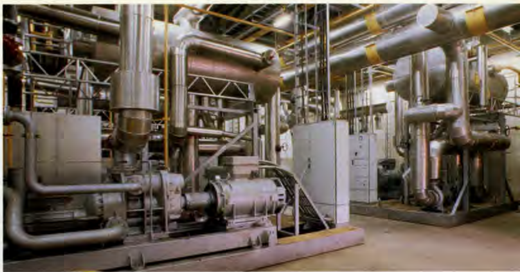
7. Energy centre, showing chiller in the foreground.
