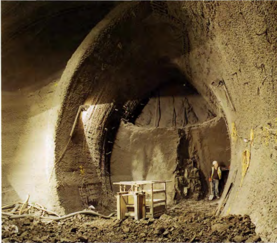
9. 8.3m diameter NATM chamber at Terminal 1, during excavation and primary lining of side wall drift.
