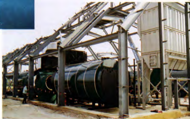
5. Installation of (left to right) flue gas diverter, waste heat boiler, and fabric filter (baghouse).
