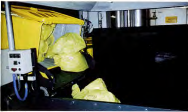
6. Bags of waste being tipped into the incinerator hopper.
