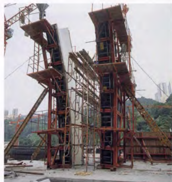
8. Wooden formwork on steel subframes used in achieving the exposed concrete finish on raking beams.
