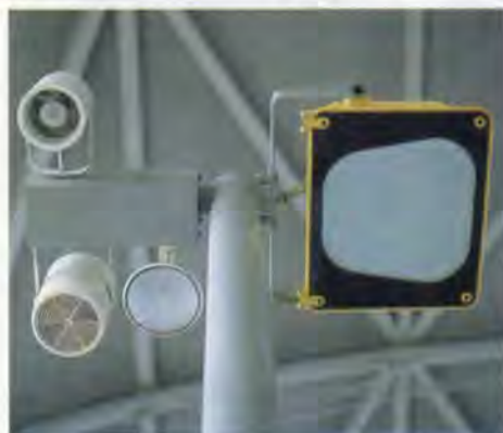
17. Technical tree: carrying fire alarm sounder (top left), public address speaker (bottom extreme left), emergency light (bottom left), light for general illumination (right).
