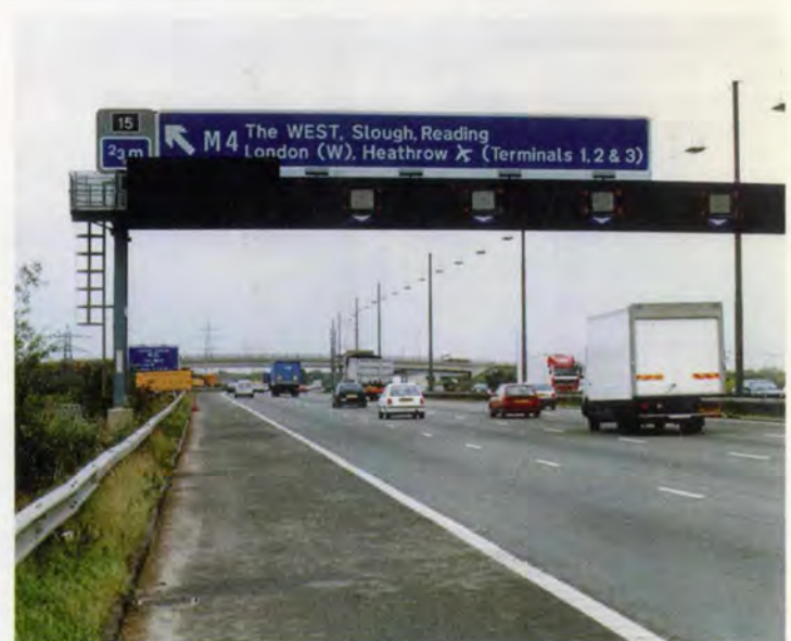
17. Typical gantry over a dual four-lane motorway, with matrix signals for lane control and a variable message sign.
