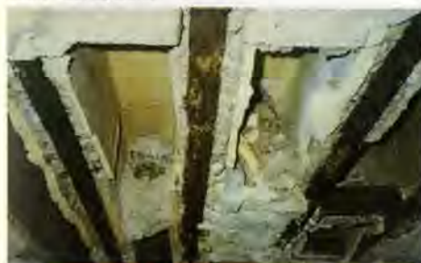
8. Concrete deterioration to soffit of Kahn floor system.
