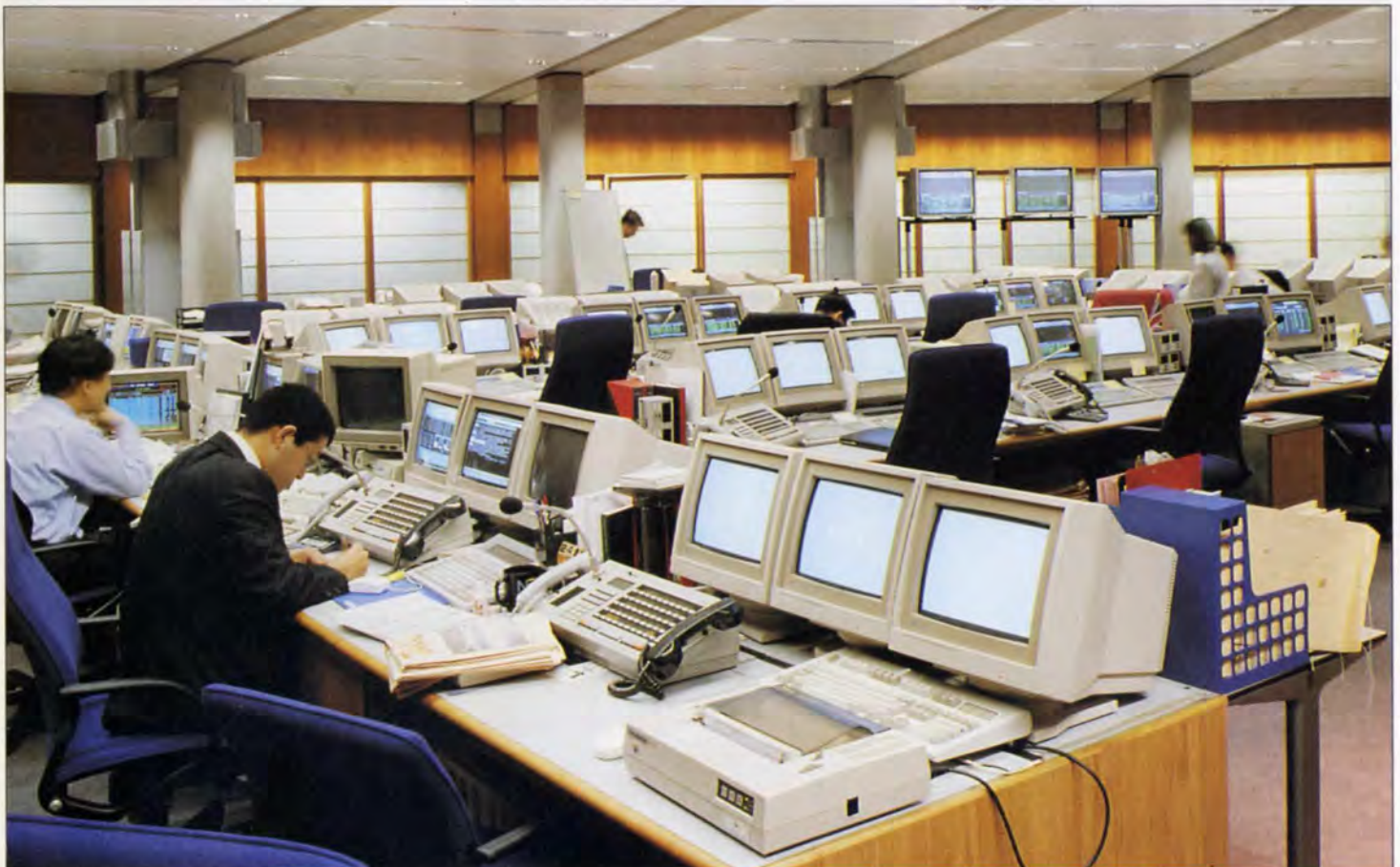
13. Completed dealing room with supplementary coolers at rear, fronting every other column.
