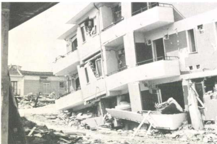
Fig.1 Strong motion damage (Italian earthquake, 1980) (Photo: R. Spence)
