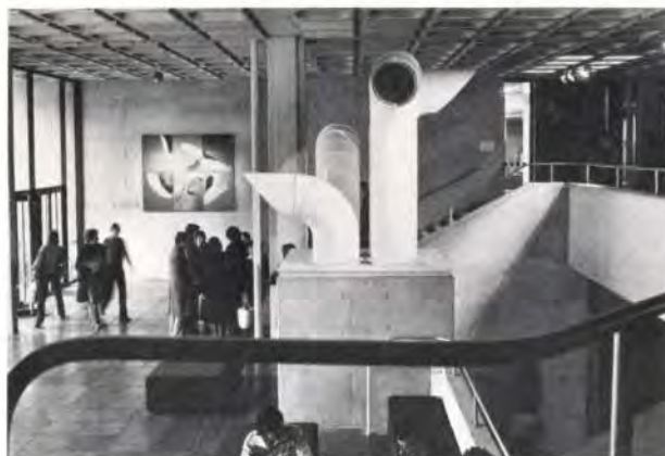
Fig. 16 The entrance hall, using air conditioning ducts as sculpture (Photo: Antoine Raffoul)
