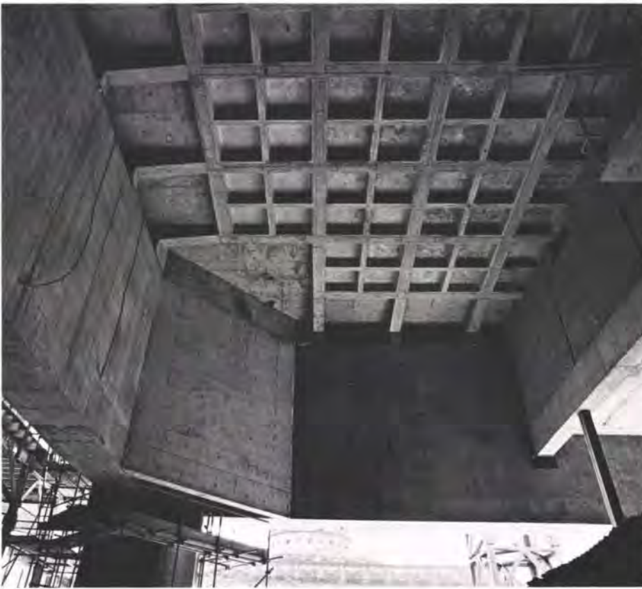
Fig. 12 Level 1 prestressed beams from within the ground floor foyer area. Foyer ceiling has not yet been installed (Photo: Ian McKenzie)
