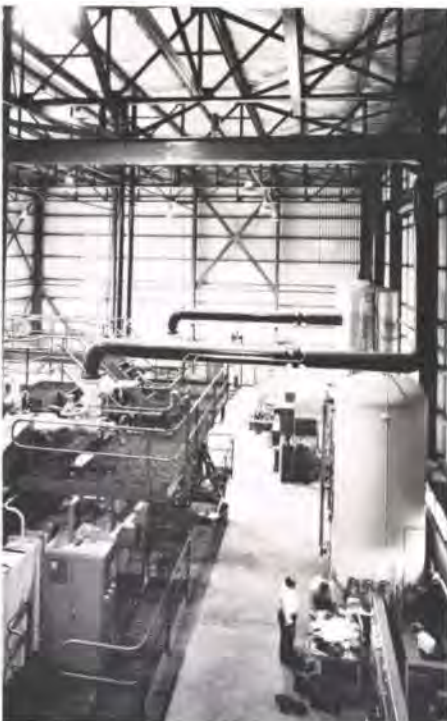
Fig. 7 Interior of the boiler house (Photo: Lincoln Harvey)
