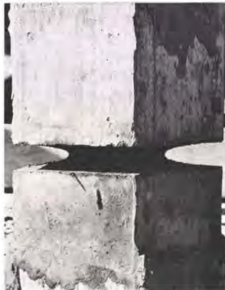
Fig. 11 Freyssinet hinge at the base of a mullion (Photo: Ian McKenzie)
