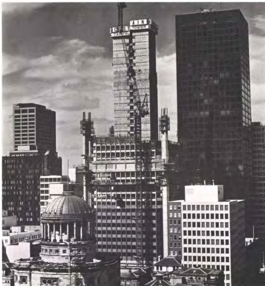
Fig. 4 Capital Tower, March 1976, from the north with the Law Courts in the foreground and the BHP building behind (Photo: Ian McKenzie)
