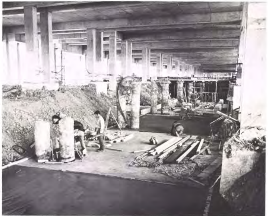
Fig. 5 Construction below Level 2, Level 0 slab being formed in the foreground with Level 1 at the rear (Photo: Lincoln Harvey)
