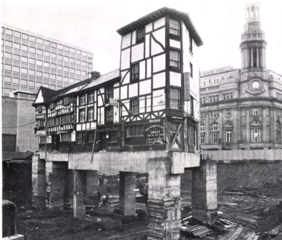
Fig. 19 View from north after main contract excavation had been completed (Photo: Stan Parkinson)
