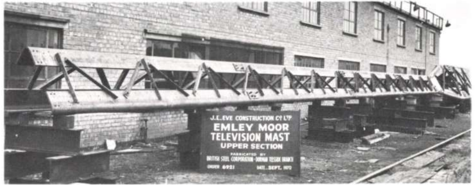
Fig. 5 right The aerial mast partially assembled during trial erection (Photo: British Steel Corporation, Teesside Photographic Unit)
