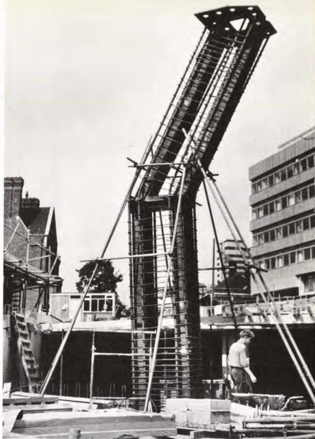
Fig. 9 Cranked column reinforcement formed by two 12 in. x 12 in. universal columns and eight 2½ in. diameter Hi-bond bars. (Photo: Peter Ryalls)
