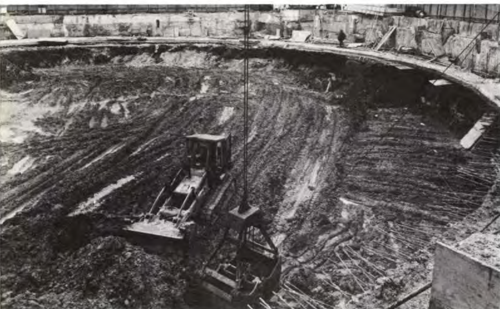
Fig. 6 Excavation of car park showing stiffening ring (cast on ground) supported by raking ties. Excavation was entirely by mechanical equipment with complete elimination of any temporary propping. (Photo: E. J. Studios). Reproduced by courtesy of Taylor Woodrow Construction Ltd., who are the main contractors.
