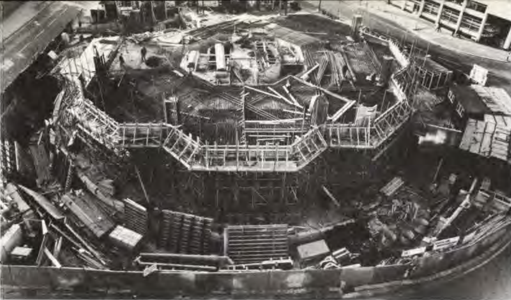
Fig. 12 1st floor level showing column reinforcement erected between 1st and 2nd floors and templates attached to the reinforcement. Some stressing cables are shown in position. (Photo: E. J. Studios). Reproduced by courtesy of Taylor Woodrow Construction Ltd.
