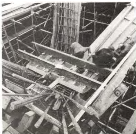
Fig. 8 above Positioning of top shutter to central support. (Photo: M. T. Walters and Associates Ltd.)
