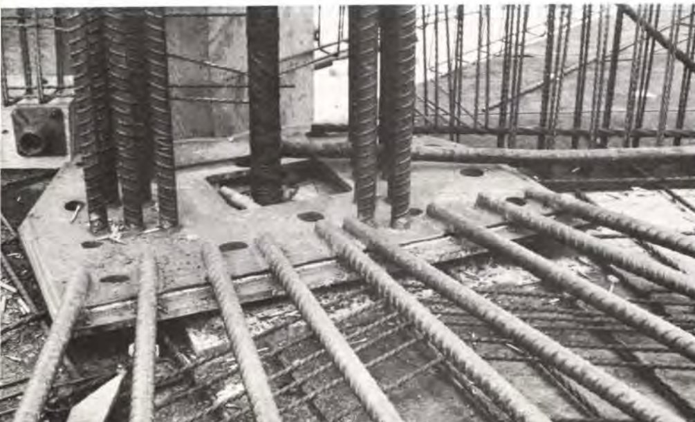
Fig. 11 Column at 1st floor level showing loose plate with 22 2 1/4 in. diameter vertical bond bars and nine horizontal 2 1/4 in. diameter Hi-bond bars welded to it, and loose plate welded to upper plate of the fabricated column. The 6 in. diameter rain water pipe is also shown passing vertically through a rectangular hole in centre of plates. (Photo: Peter Ryalls)
