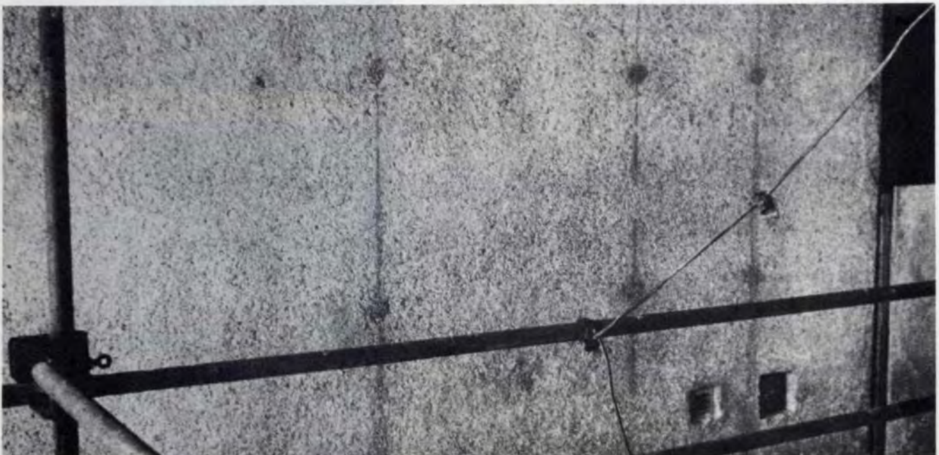
Fig. 4 below Tower Block 1. Staircase wall after bush-hammering; shutter joints and bolt holes still show
