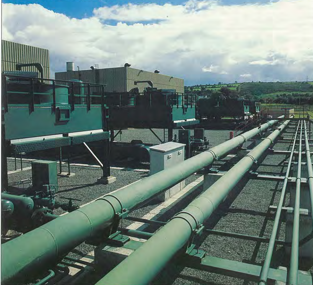
9. View from north west showing main headers and fin-fan coolers.
